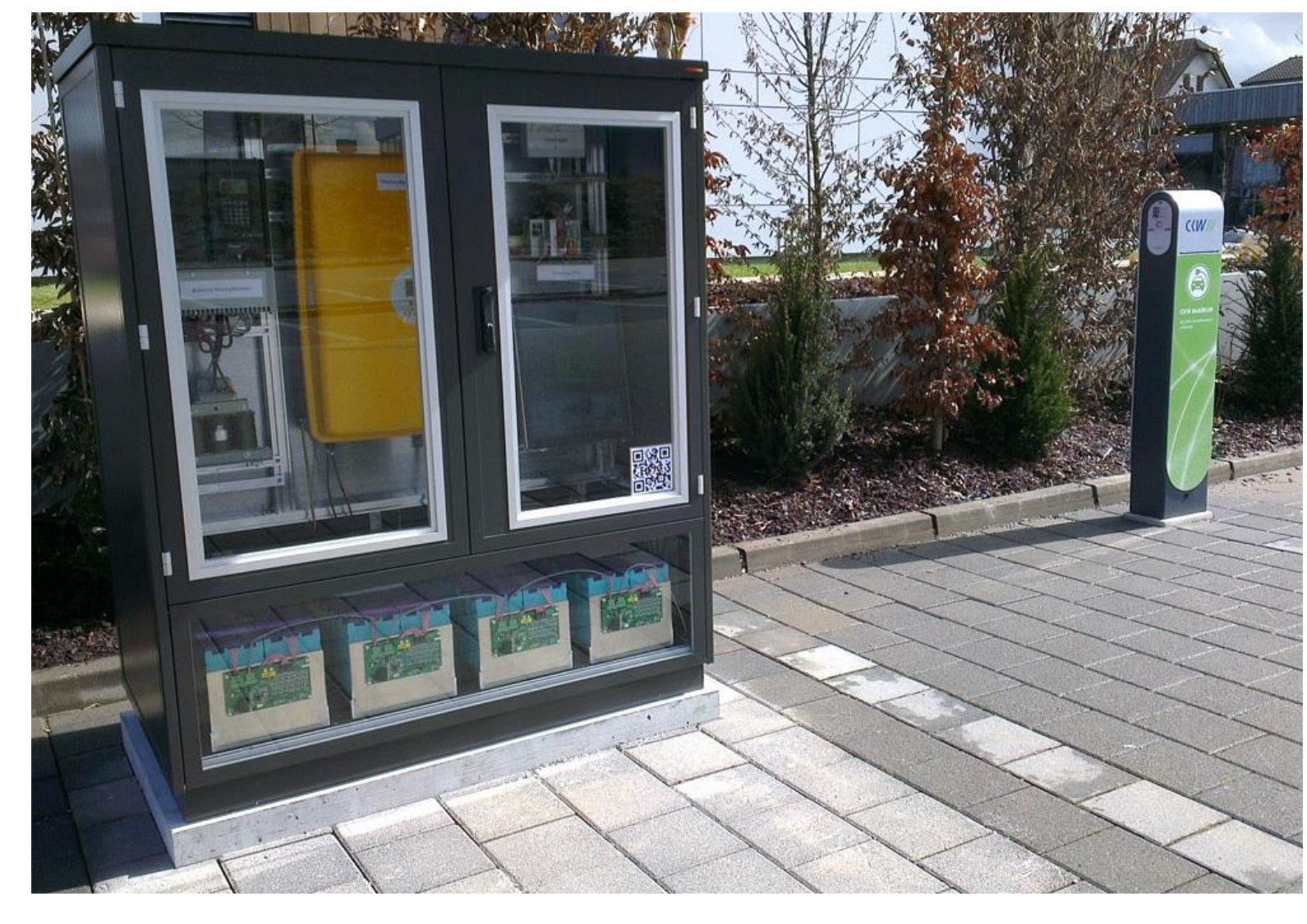
Stationary Smart-Grid Storage
